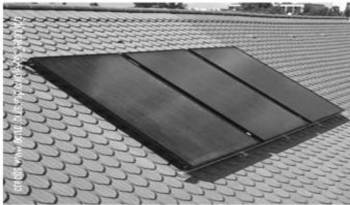
Fig 1. Glazed flat plate collector
