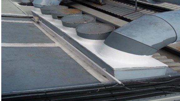
Figure 1: Example of erosion-corrosion on HVAC system components. Source: [Smith & Brown, 2019].
