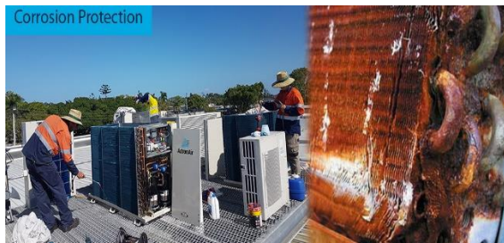
Figure 1: Corrosion impacting your HVAC Equipment Performance
