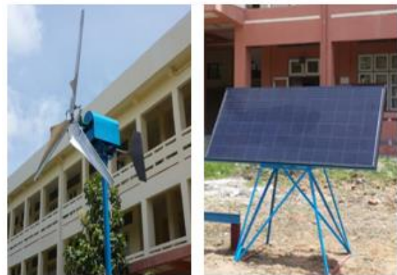
Fig.1. Project Photo of Wind Turbine and Solar Panel
